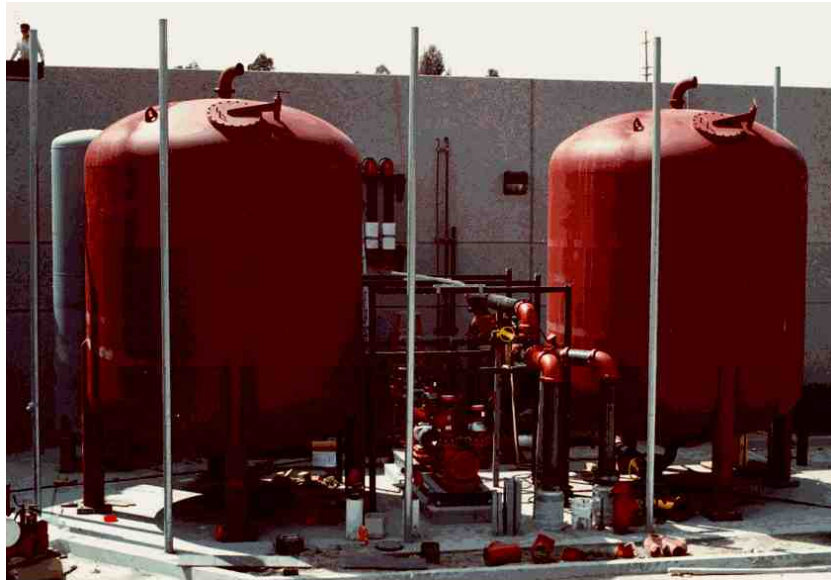
Cryogel Ice Ball system, exterior TES-Ice installation
